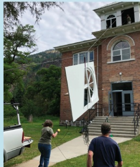
...we helped restore the bell tower on the Paradise School in Sanders County.
