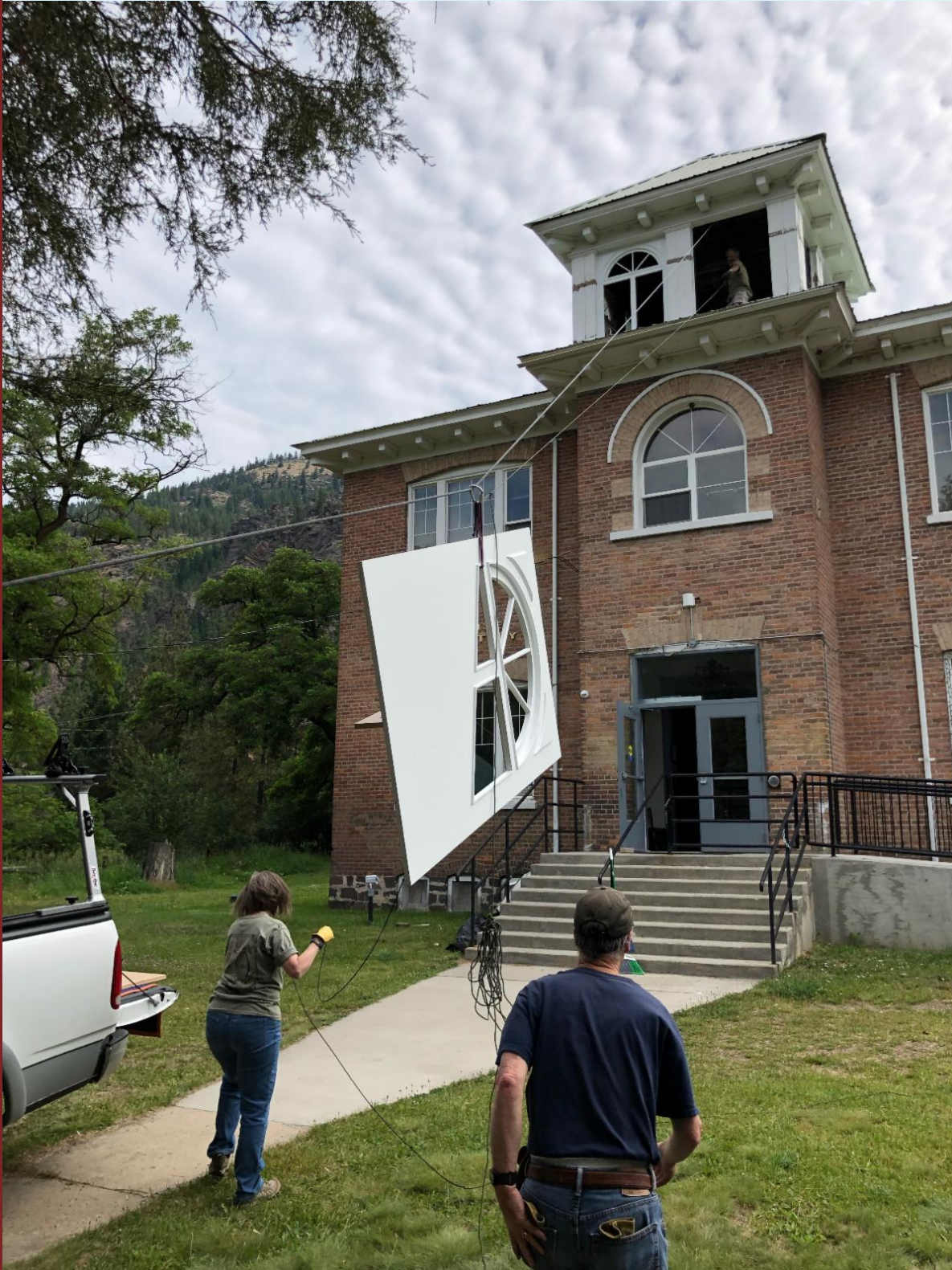
2019 grantee Paradise Elementary School Preservation Committee works to repair the historic bell tower, which is home to the original school bell cast in 1886.
